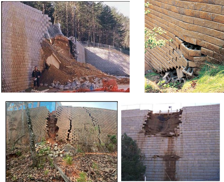
Figure 1 MSE Walls failure due to hydrostatic pressure and rainfall
