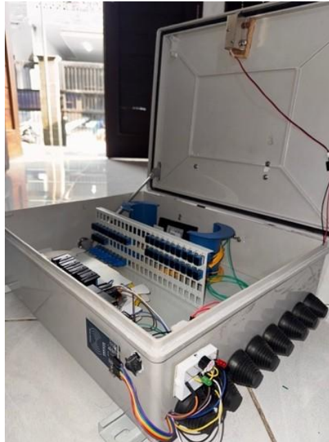
Figure 10. Implementation of Auto Lock System Prototype on ODC Prototype
